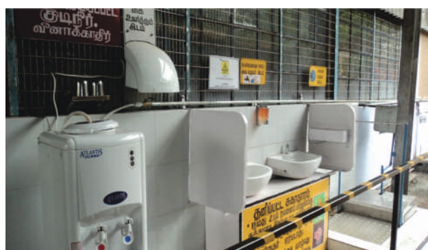
Wash station at main entrance
